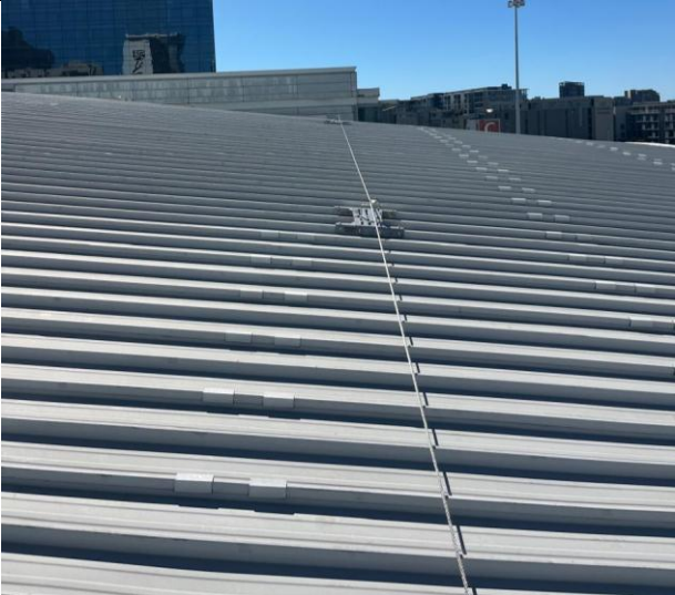
Safe Walk Fall Arrest System, located on the Roof of CTICC 1
